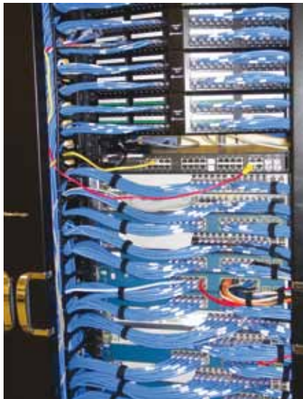
Figure 1. A well-installed, well-structured cable enclosure using color-coded cabling makes for a much more professional appearance and also demonstrates adherence to specific standards.
